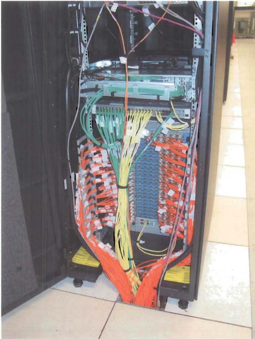
Figure 2. RoadRunner Node Cabling
