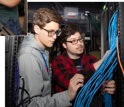
Interns cabling their mini-supercomputer.
